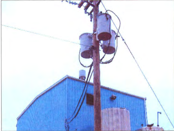
Pole mounted transformers located at the Custom Chemical facility.
