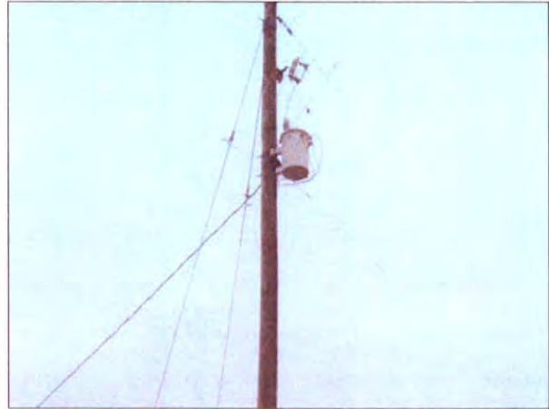
Pole-mounted electrical transformer located on the subject property
