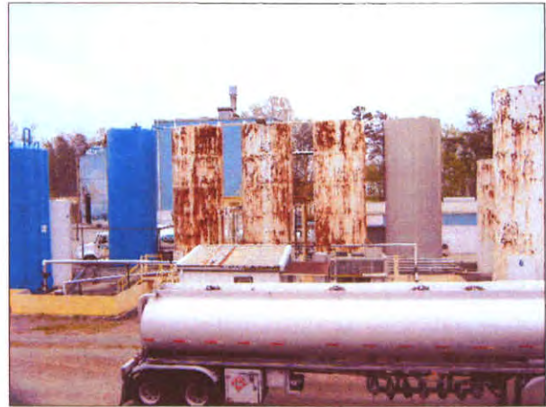
Vertical ASTs located on the western side of the Custom Chemical facility – note the condition of the ASTs.
