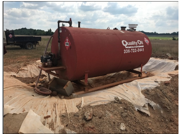
Diesel AST in the area of the active construction
