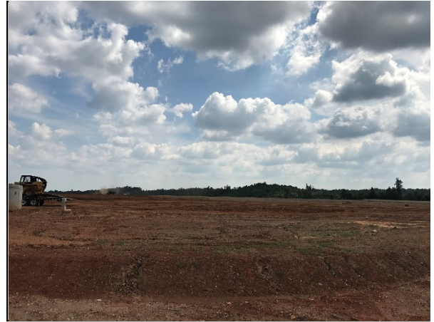
Eastern view from the active construction area in the northern area of the Site
