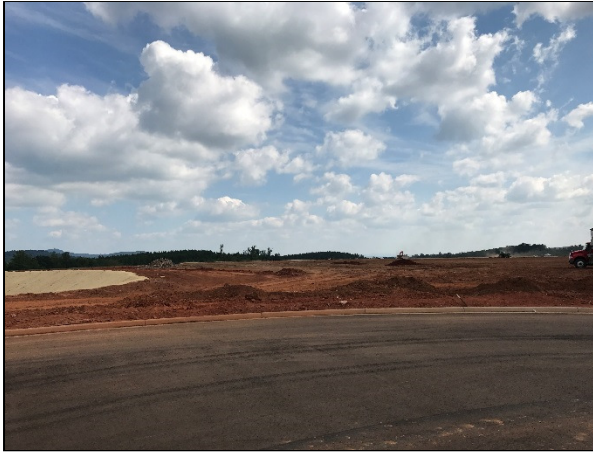
Eastern view from the active construction area in the northern area of the Site
