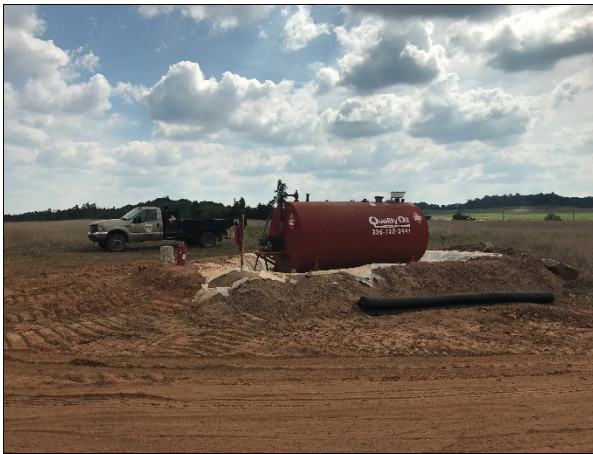
Diesel AST in the area of the active construction
